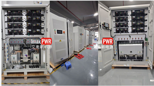
30 × 500 kW PV+storage cabinets
