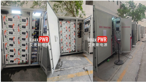
12 × 125 kW / 261 kWh systems
