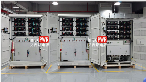
1.5 MW PV+storage cabinet
