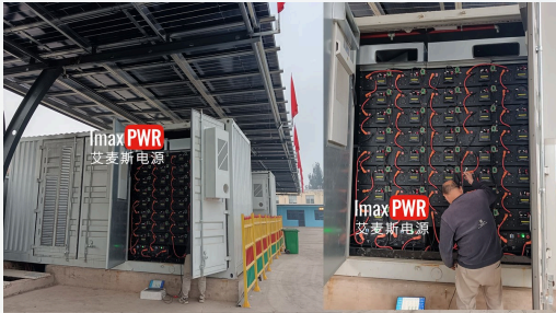
3 MWh ESS cabinet
