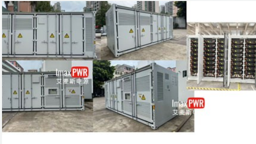
1.7 MWh ESS cabinet
