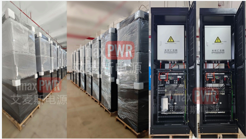
36 × PV control cabinets
